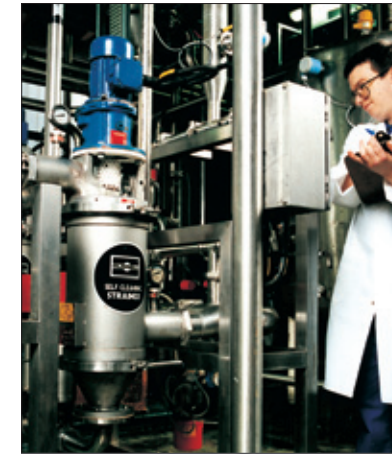
Self-Cleaning Russell Eco Filters® provide pre-filtration at a factory of H.P. Bulmer - Cider manufacturers
